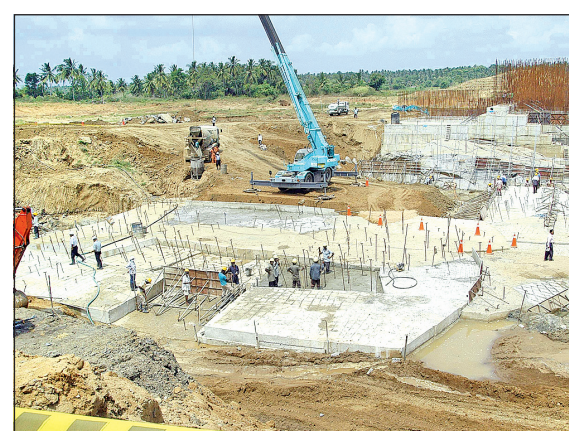
The Deduruya Oya project to bring thousands of lands in the North Western Province under the plough.
