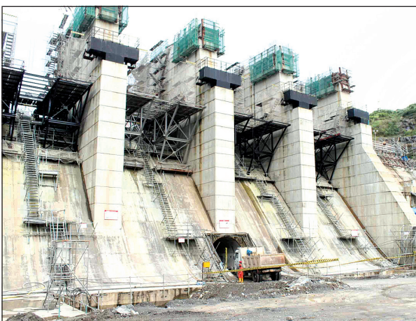
The Upper Kotmale project - mega scale hydro power generation project in the country
