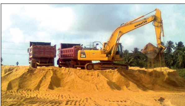
Construction work on the Katunayake Expressway connecting the Bandaranaike International Airport with Colombo and other cities is in progress.
