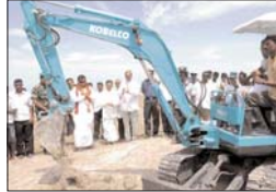
A new water supply project being commissioned in Delft island
