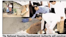
The National Housing Development Authority will construct 328 houses islandwide to mark President Mahinda Rajapaksa's second term in his office. Here Minister Wimal Weerawansa lays foundation for the first house in Ranala Kaduwela. Picture by Ashraff A Samad Dohwela-MI Lavinia Sp Cor
