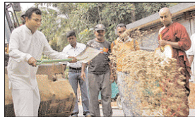
The rehabilitation of a long neglected road, M. D. H. Jayawardhana Mawatha, Aturugiriya was started recently by the Western Province Road Development Authority under the direction of the Education Minister Susil Premajayantha and Western Provincial Council member Deshabandu Jagaththama Liyanage. Here the residents of the area who also participated in the work with the Chief Incumbent of the Seewali Asapuwu temple Ven. Padalangala Dhammaveera Thera and Principal Oruwalla Vidyalaya Amarasing Devasa. Picture by Dushmantha Jayadana
