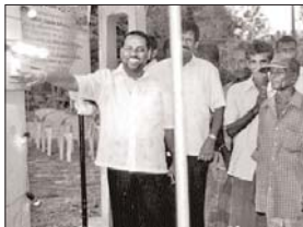
Dr. Haris Deen from Doha, Qatar and Presidential Advisor Hafiz Nazer Ahmed laying the foundation stone for the new building of Kuliyathul Dhariul Uloom Arabic College, Eravur.
