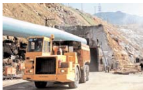
A heavy vehicle and the huge ventilation tube at the entrance of the access tunnel to the head race tunnel at the dam site in Thalawakelle.
