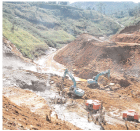
The construction site of the proposed dam across Kotmale Oya, near Thalawakelle Town, is one of the major civil construction works with heavy machinery buzzing, excavating the dam foundation.
