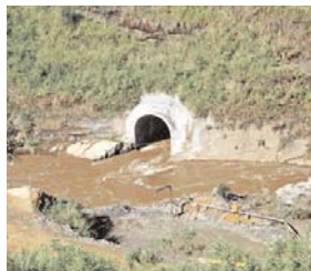
Waters of Kotmale Oya enters the 300 m long diversion tunnel at the dam site.
