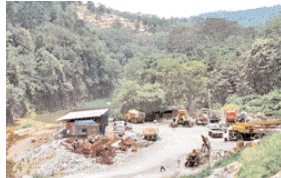
The waters of Kotmale Oya after producing electricity meets the upper reaches of the existing Kotmale Reservoir at Niyangamdora power house site.
