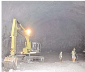
A backhoe shaping the inside of one of the access tunnels carved into granite rock. The access road facilitates the construction of a 12.5 km long main tunnel or the head race tunnel which carries water from the reservoir at Thalawakelle to the power house at Niyangamdora in Kotmale.
